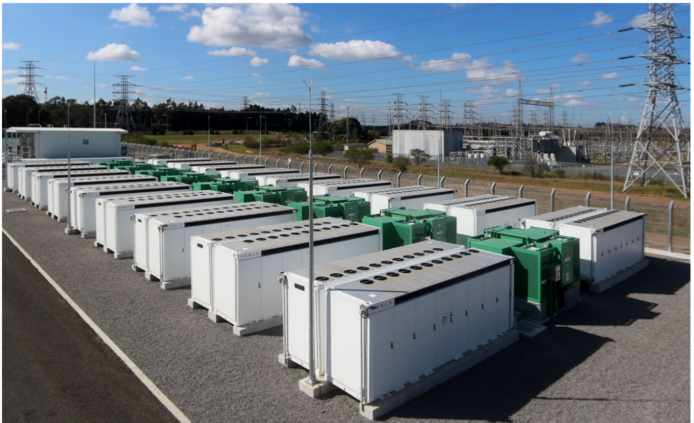
Photo 2 – Wallgrove Grid Battery looking towards Sydney West substation
