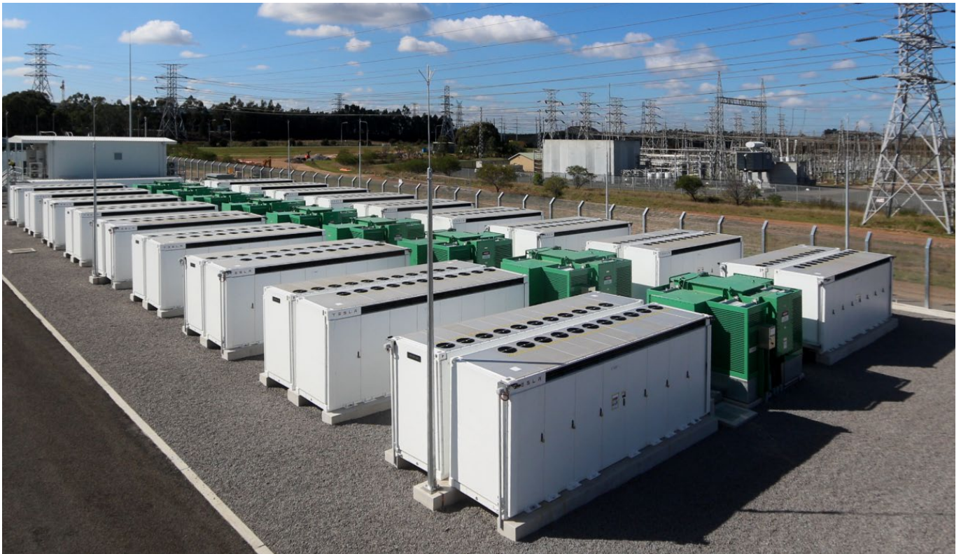
Photo 1 – Wallgrove BESS looking towards Sydney West 330/132kV Substation
